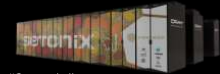
“Setonix” Pawsey Supercomputing Ctr, Australia
