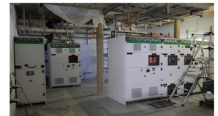
low voltage switchboard 2025 HPC USER FORUM
